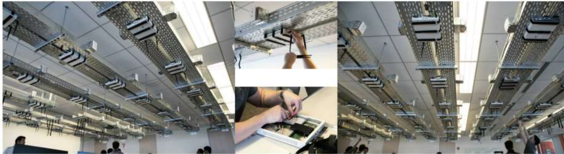
Fig. 2. VT/CCI xG Testbed. With 72 nodes, 4 MEC, and O-RAN capability, this is one of the largest university-based SDR testbed in US.
